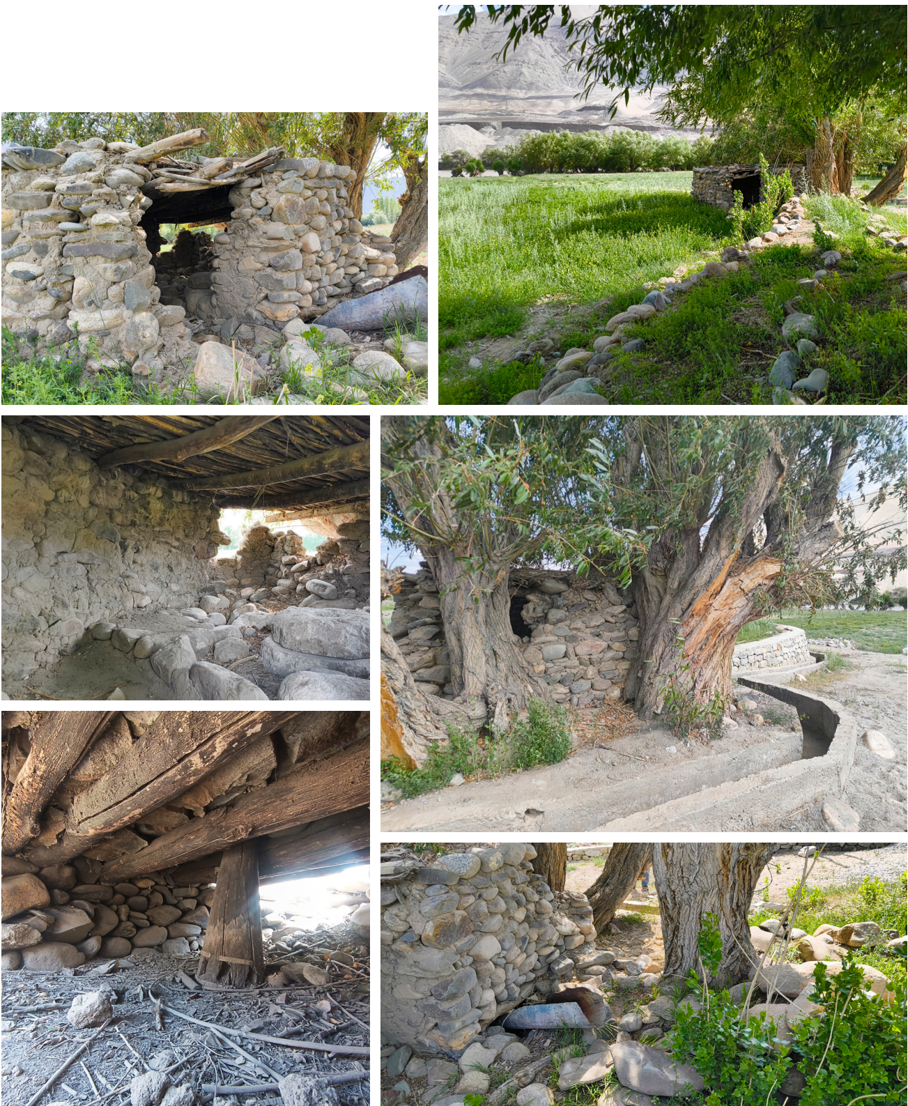
First row: Elevated water channel ( wato ) originally designed to divert flow from the nearby stream to the rantak. Entrance of the old rantak, with the door missing and lintel fractured.
