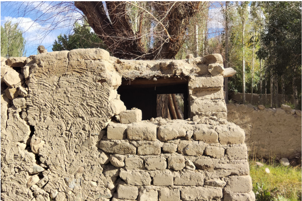
The rantak's corner collapsed, exhibiting pronounced diagonal cracking on both sides. Images: Field Studios
