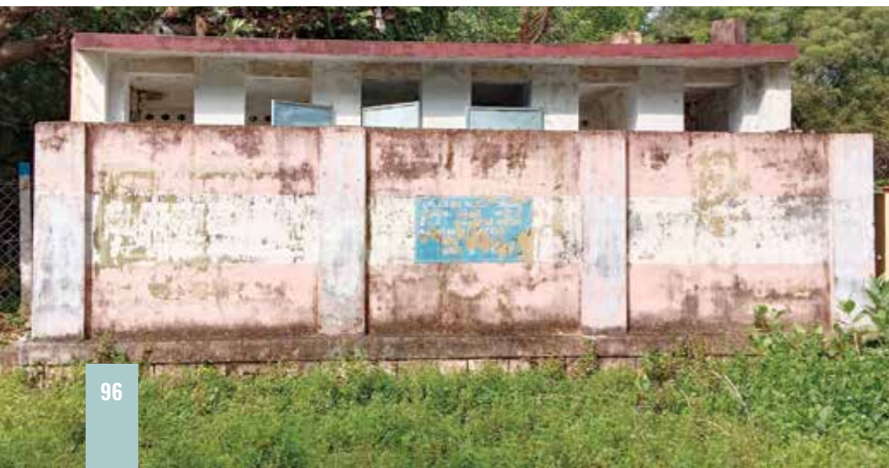
Non-functional community toilet located near the river in Thirupudaimaruthur hamlet.
