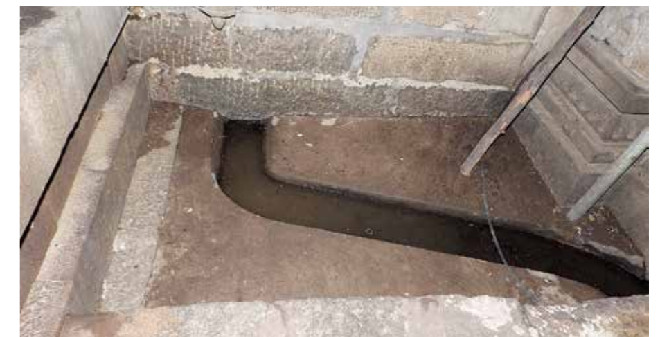
Stagnant water and uncovered drains within the temple premises.
