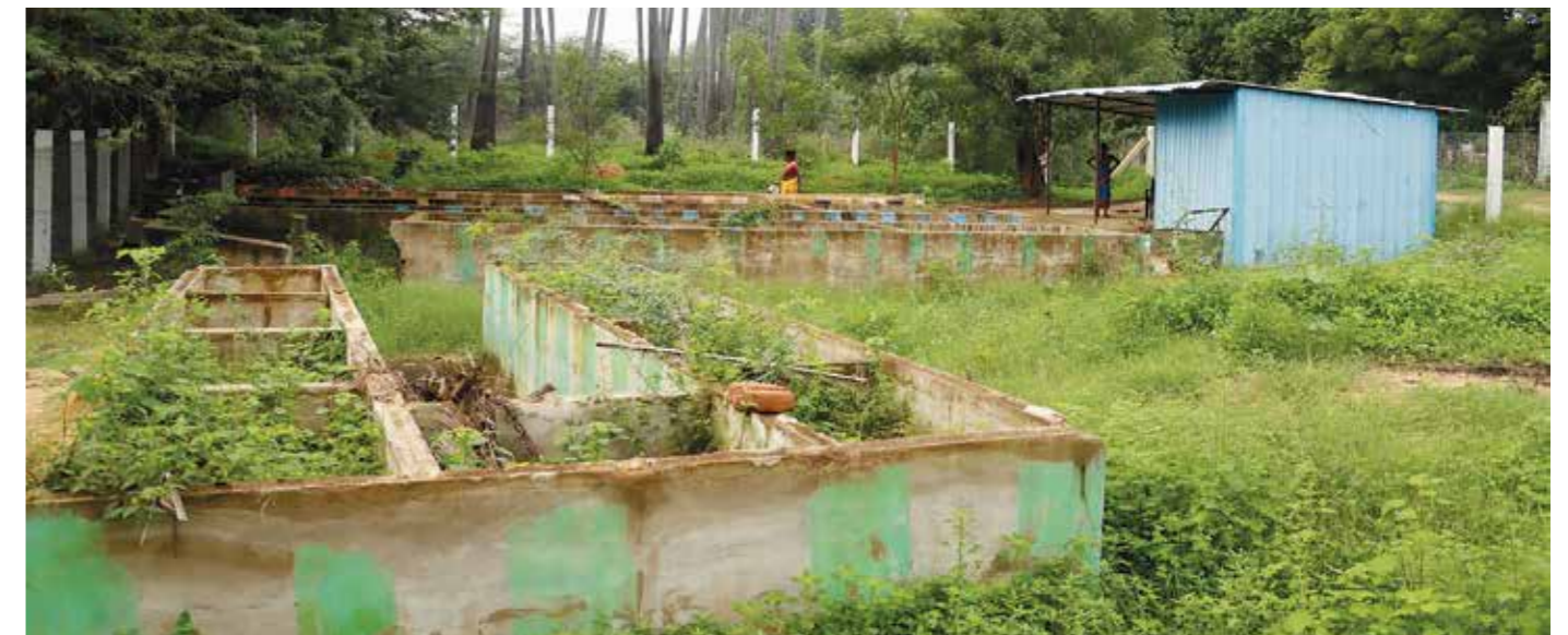
Dilapidated waste segregation facility located in Thirupudaimaruthur.
