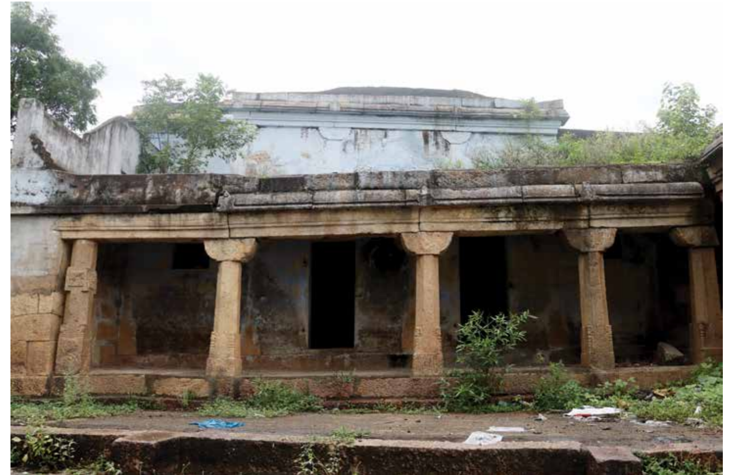
Changing rooms near the the river in a dilapidated condition
